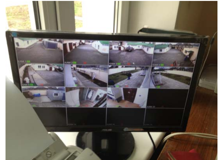
The installed video surveillance cameras.
